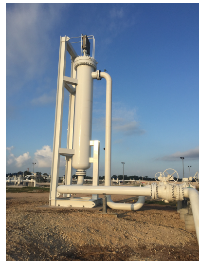
A previous installation of a single vessel AOT unit on a commercial pipeline.
