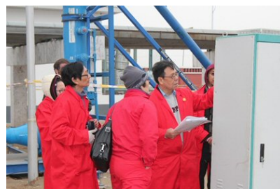
Dr. Rongjia Tao, chair of the Department of Physics at Temple University, conducting viscosity reduction testing of an AOT prototype installed on a commercial pipeline located in PetroChina's oilfields near Chaoyanggouzhen, China.
