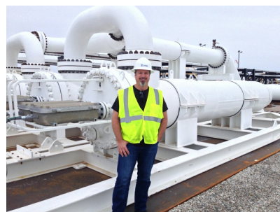
A field AOT installation with John, a QS Energy Project Manager
